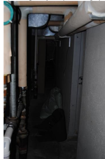
Plumbing & ventilation between cell blocks
