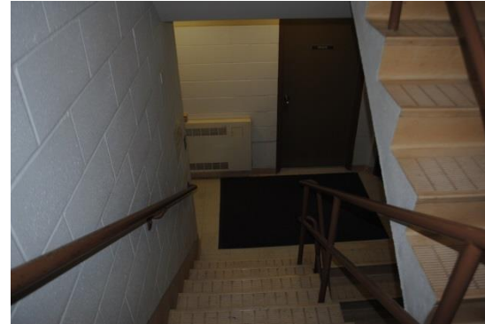
The stairway from the outside door to the SA Office. The primary security concern is related to the office's entrance. There are no cameras in the hallway. The office area is separated by a wooden door with a security keypad, which is left unlocked during business hours.
